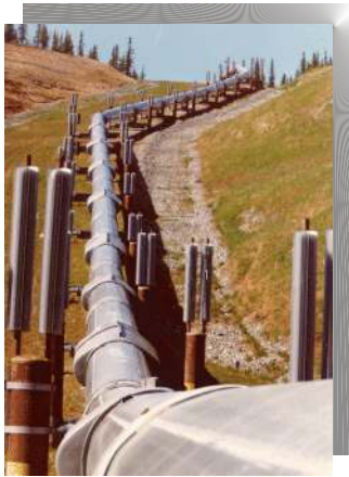
48 inch Trans-Alaska oil pipeline
