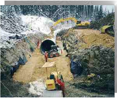
Suncor Energy - Wilkie Creek Culvert Replacement Incorporating Rock Drops Inside Culvert for Fish Passage, Alberta - 1998
