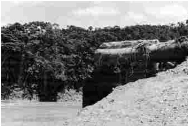
Trans-Ecuadorian pipeline (SOTE) severed by flood water, east bank of the Aguarco River. ("The March 5, 1987, Ecuador Earthquakes, Mass Wasting and Socioeconomic Effects". Natural Disaster Studies, National Research Council, 1991).
