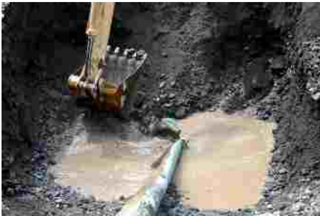
Rio Reventador, Damaged OCP Pipe due to May 5, 2003 Flood
