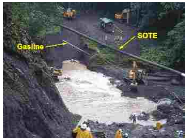
Construction of Rio Reventador crossing complicated by proximity of existing high pressure lines.
