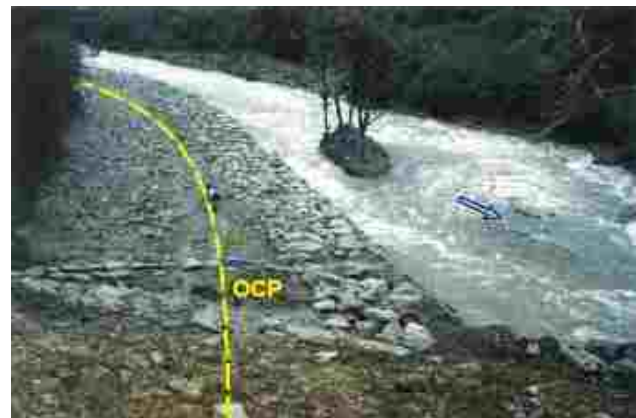
Instream section in upper reaches of Rio Papallacta. Pipeline protected by cover depth and riprap.
