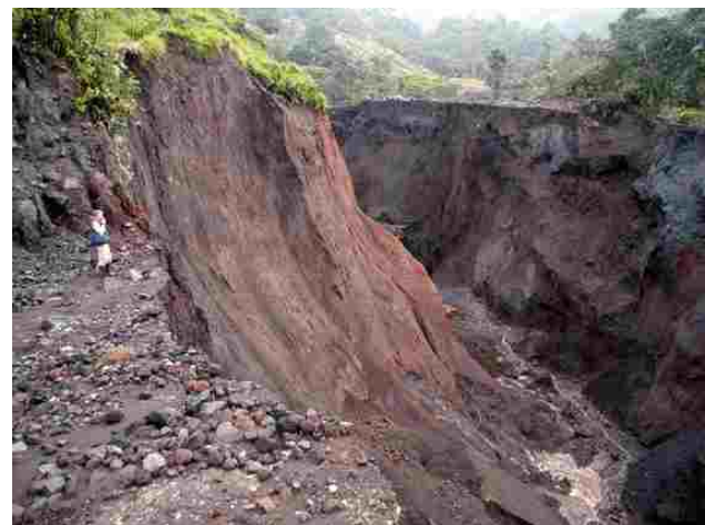
Erosion of Main Highway as a result of overflow from Rio Reventador. Note man at left for scale.
