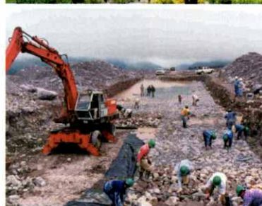
Top: the pipeline passes through narrow and steep rights-of-way through the mountains. Above: local labourers help place a 57-metre, one-metre thick gabion mat over the pipeline as protection.
