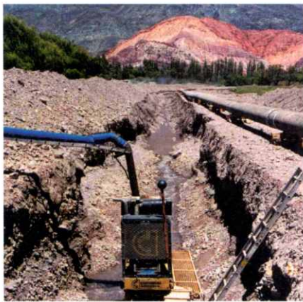
Excavating a ditch for the pipeline in Rio Purmamarca. The riverbed was restored and steps were taken to protect the small irrigation systems of local farmers.
